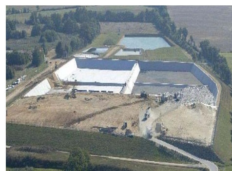
Figure 5 : Photo of the bioreactor cell after its filling (part recovered by earth) and of the test cell in the course of filling
