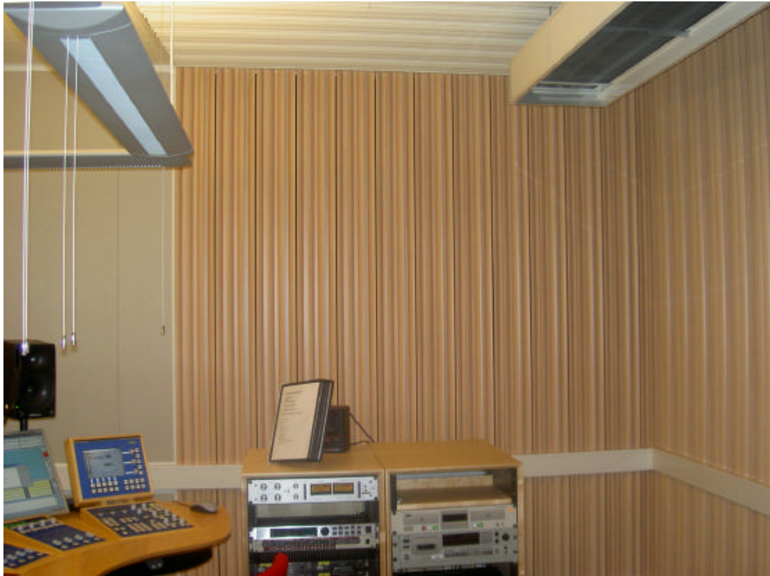
Figure 6.9. The non-preferred room, control room aspect, side view showing Ecophon Wall panel to the left. In the middle and to the right of the picture, Svanå miljöteknik AD10 diffuser panel is mounted. Note that AD10 panel is also mounted in the ceiling.
