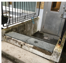
Worn out staff entrance.
