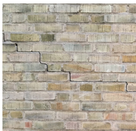
A crack in the entrance façade.
