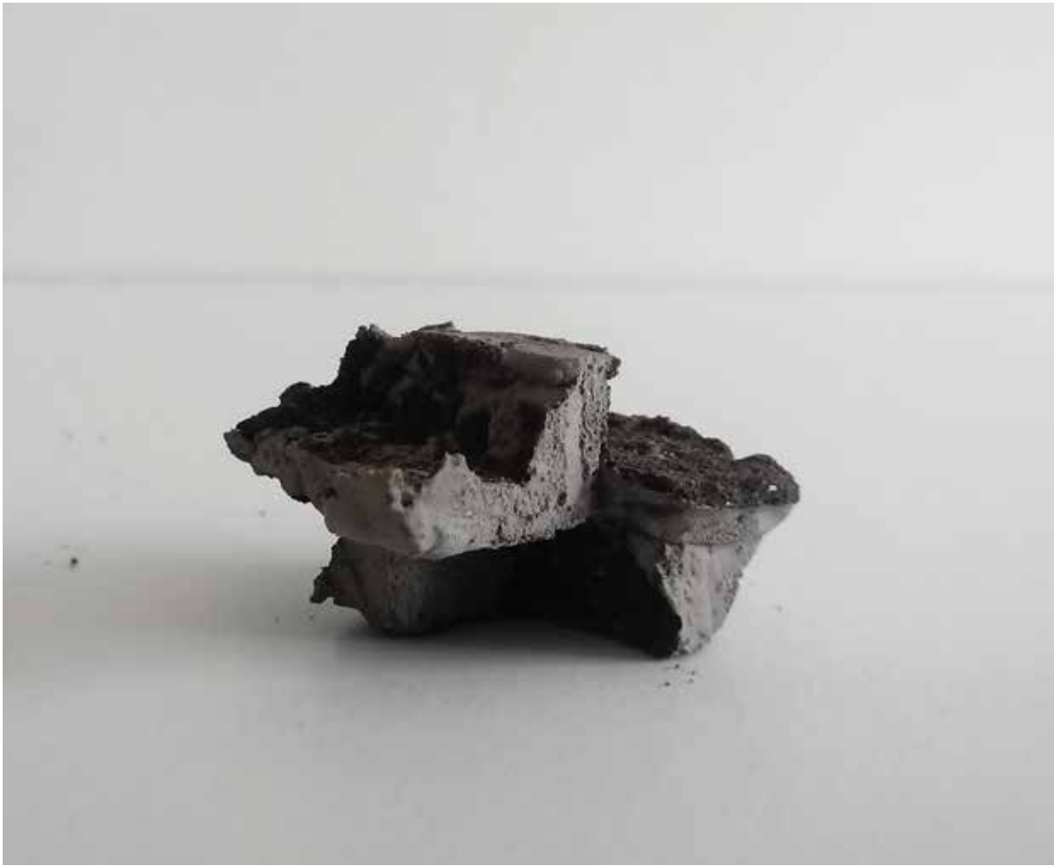
Mortar after bricks being washed away
