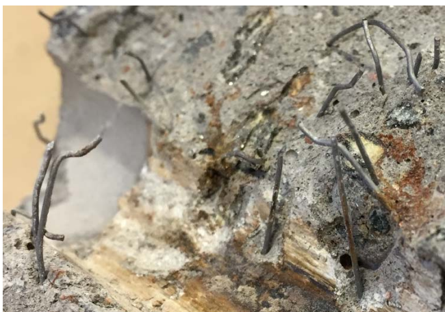
Figure 6: Example of embedded fibres located near the rebar revealing light corrosion.
