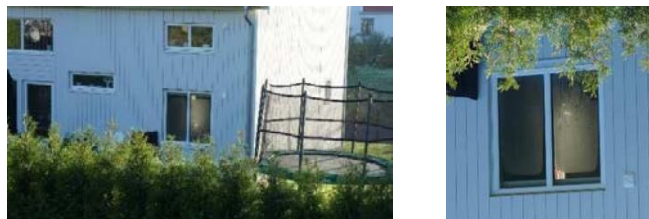
Fig. 4. Condensation on the external glaze pane of a window (photo K. Pietrzyk).
