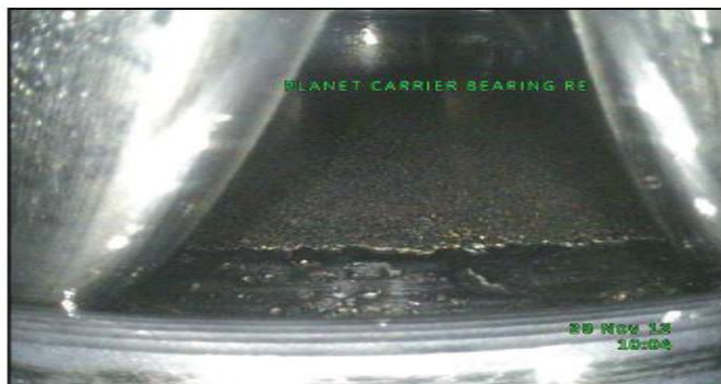
Figure 4-28 Turbine A1 bearing damage due to spalling (Adopted from WT service report)
