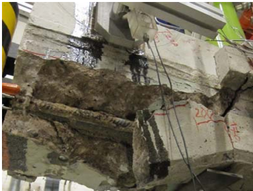
Highly damaged H2
