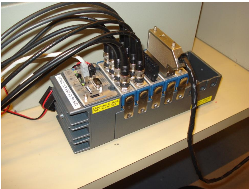
Figure 63: View of the compactRIO system.
