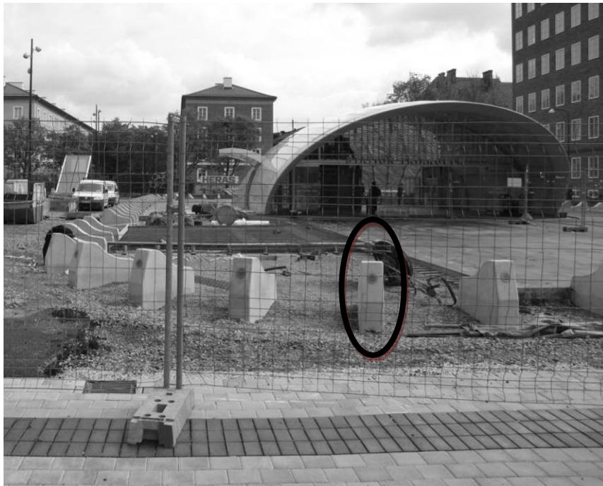
Figure 2.2. Collision protection at one of the entrances to the station Triangeln. The area around the entrance is under construction. (Photo: Cecilia Wideman)
