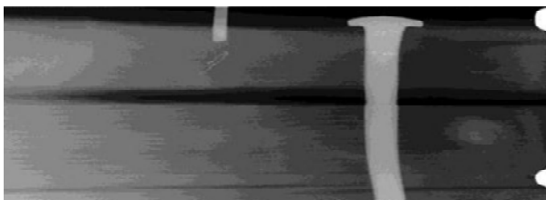
Figure 2: Clear deterioration of the metal fastener due to corrosion in the shrinkage crack of the beam [3].
