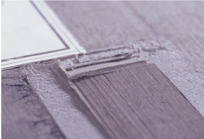
Fig. 18. Example of delamination of a CFRP laminate bonded to a steel member.
