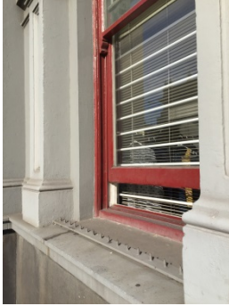
This is a window in with anti-homeless spikes (Melbourne, Australia).
