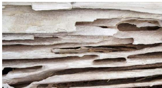
Figure 22: Termites attacked the wood.
