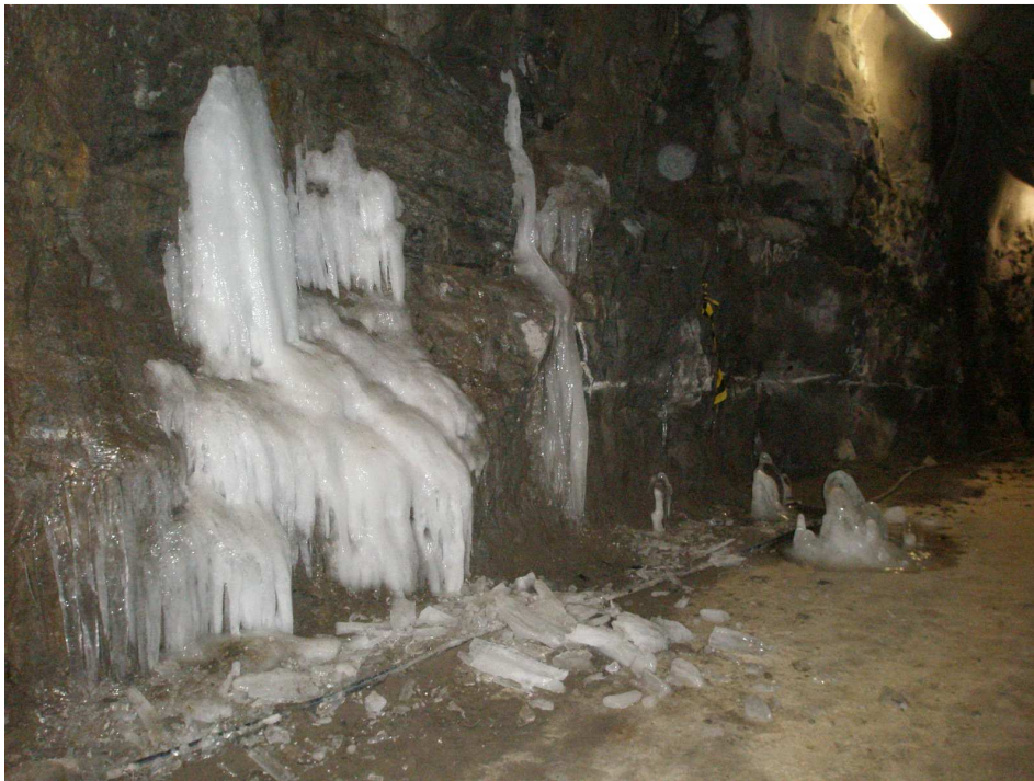
Figure 6 Frozen leakage water from fractures in bedrock in a tunnel under construction. The photo is taken close to the tunnel entrance. Photo: COWI AB.
