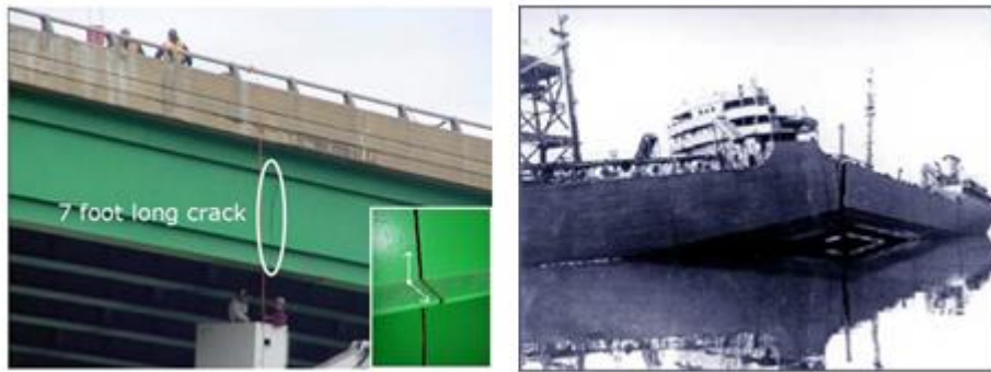
Figure 2.10 a) Fatigue crack in a bridge construction (Haghani et al. 2012) b) Fatigue failure in a ship (TWI 2015).
