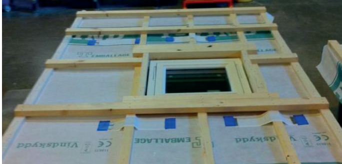
Figure 30. Indicators were positioned just below all details in the ventilation gap and behind the façade; test item A with vertical façade panel.
