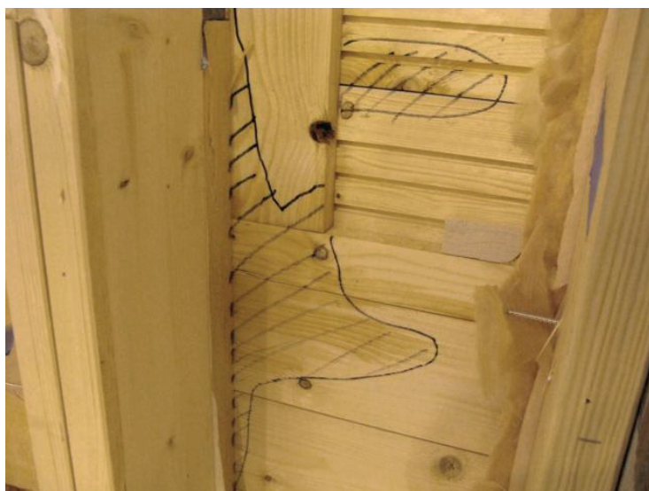
Figure 32. Photo of the back of the wooden façade panel (test item B) after the wall was opened from the inside. Highlighted areas indicate wet areas behind the façade/horizontal panel, battens and underlay board for the horizontal metal plate.
