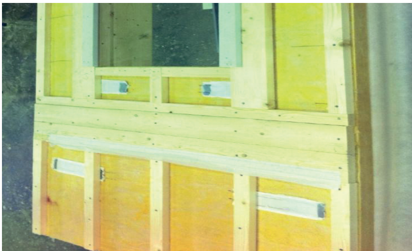
Figure 31. Indicators were positioned just below all details in the air gap and behind the façade; test item B with horizontal façade panel.
