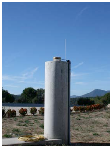
Fig. 3. Cebreros (CEBR) GNSS receiver installed in its monument.
