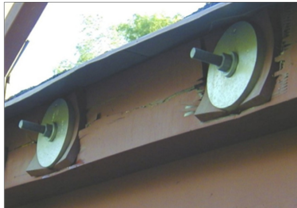
Figure 6.1 Local crushing of the timber perpendicular to the fibre direction of the edge beam. Photo taken from (Pousette and Fjellström 2004).
