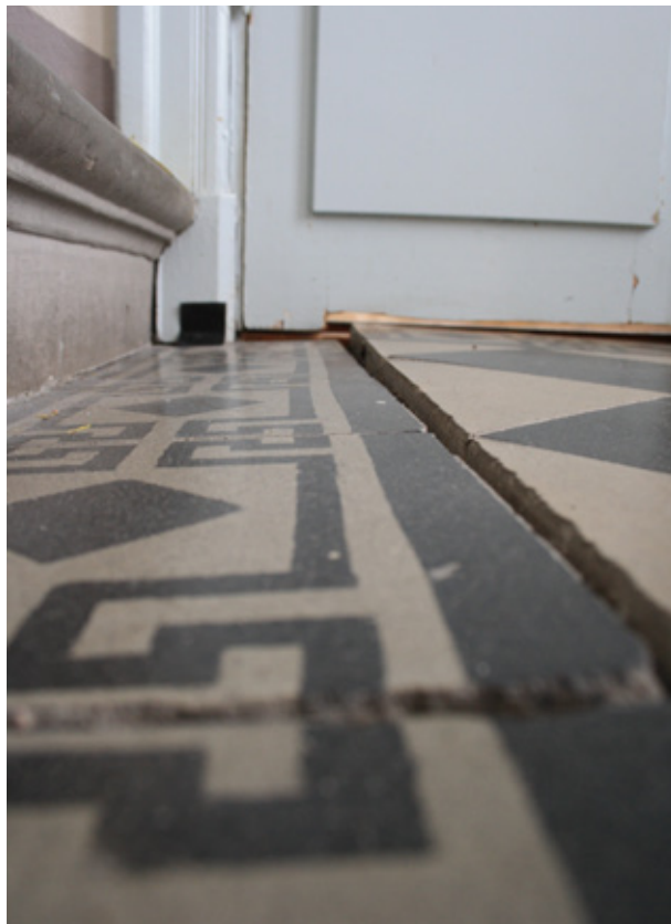
The building suffers from subsidence problems which can be seen both in the interior and the exterior
