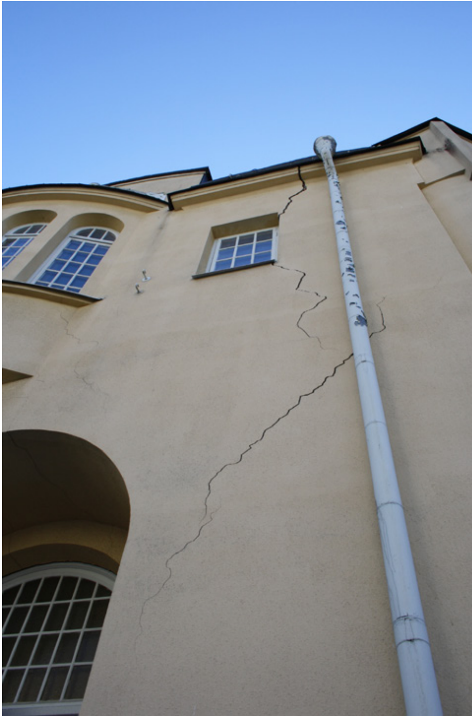
Cracks in the facade due to the subsidence damage
