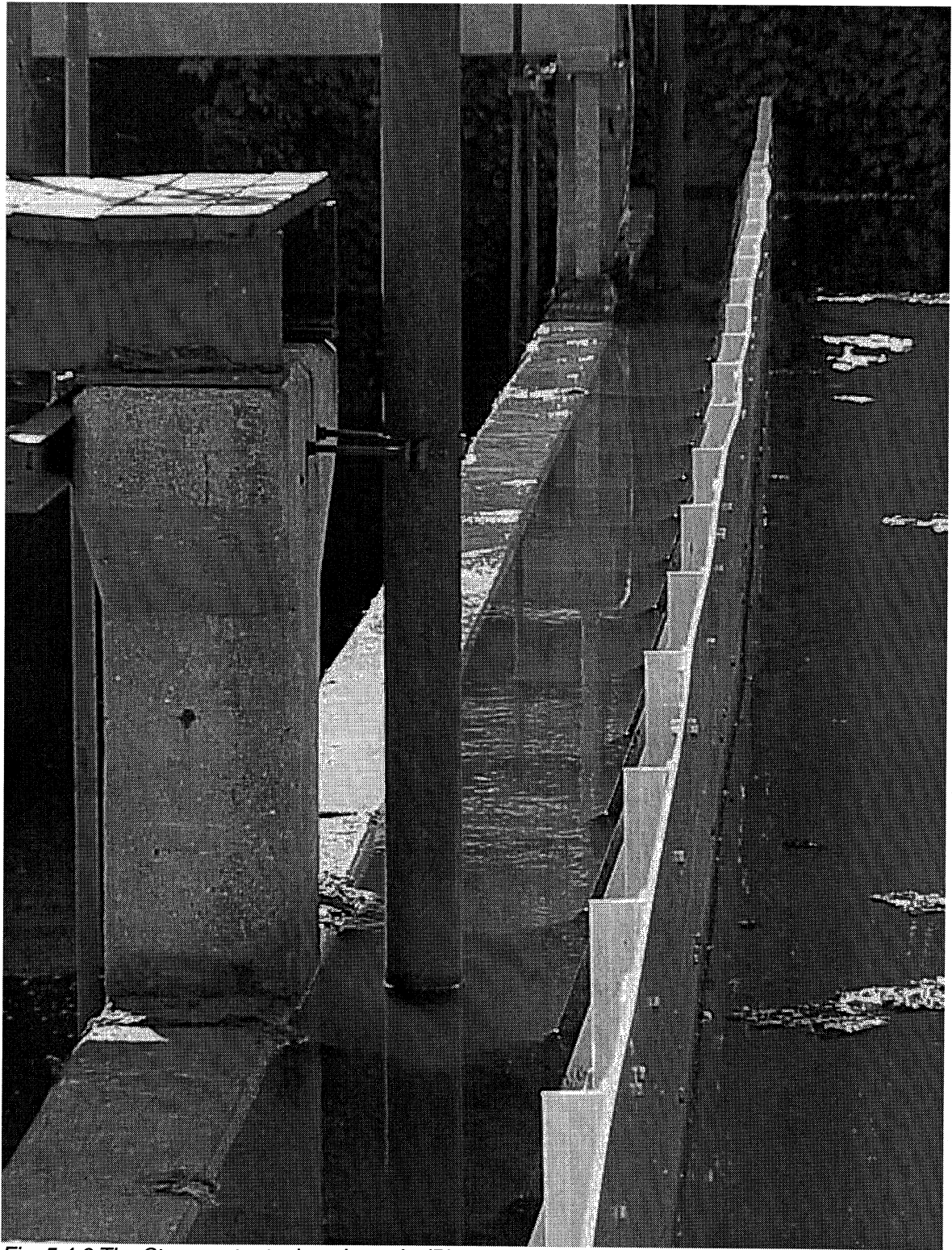
Fig. 5.4.6. The Storm water tank outlet weir. (Photo by Quintin Rochford)
