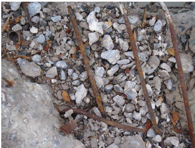
Figure 9.44 Detail of the damages at the side A test points L7M1 and L8M1.
