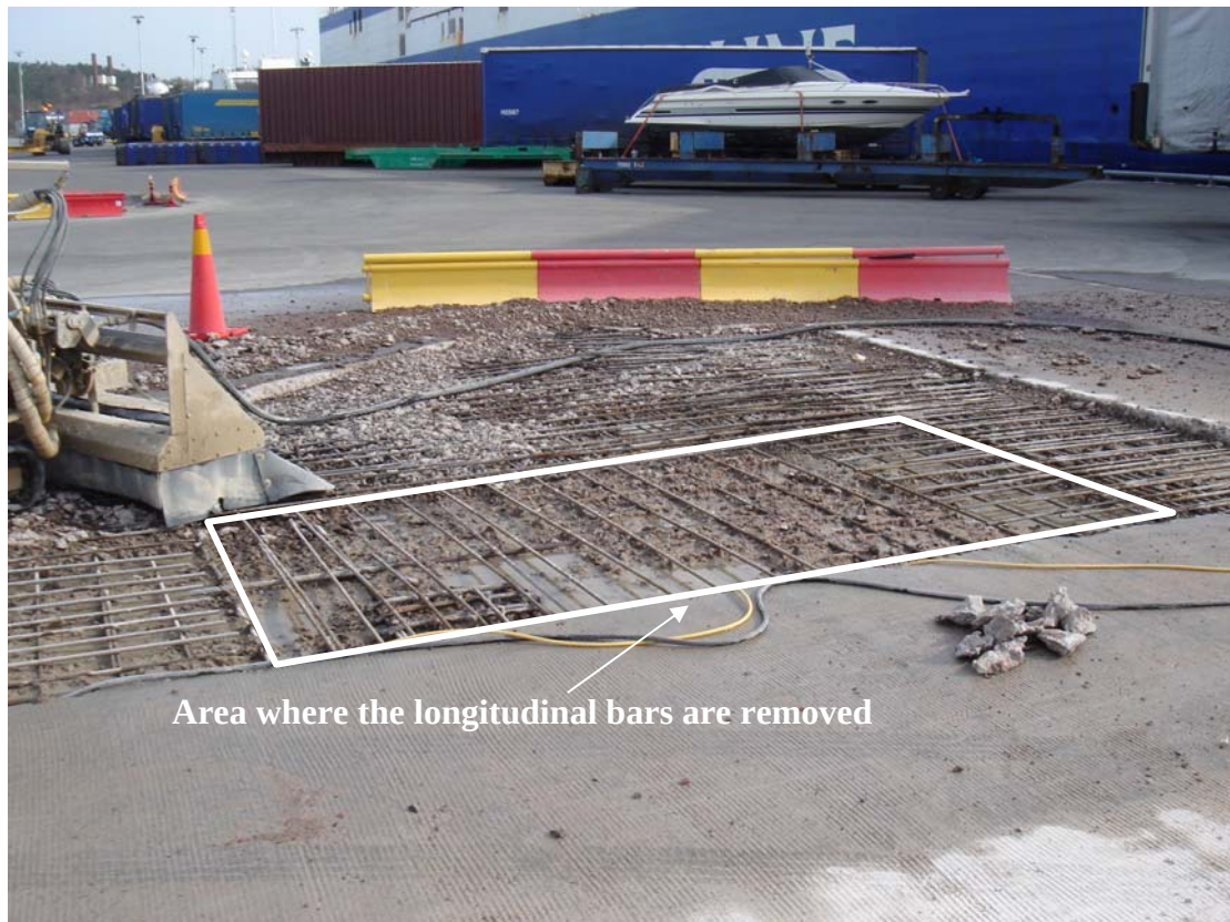
Figure 9.19 Surface 1 with some bars removed because the waterblasting process.
