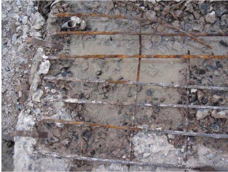
Figure 9.43 Detail of the damages at the side A test points L6M13 and L6M14.
